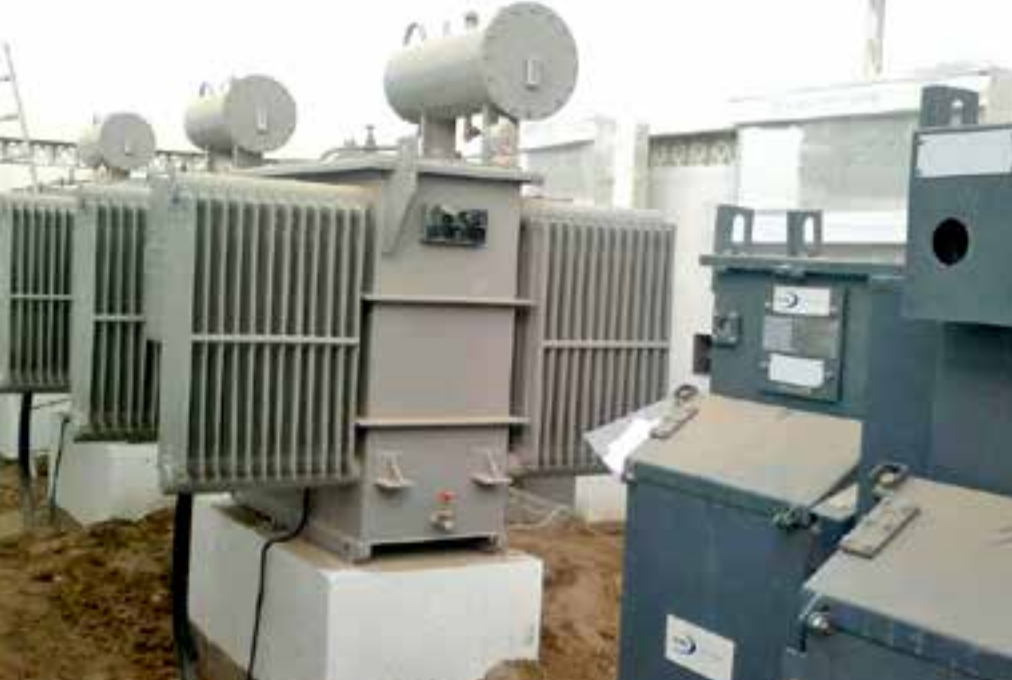
3 Nos of 1000 KVA substations with RMU
