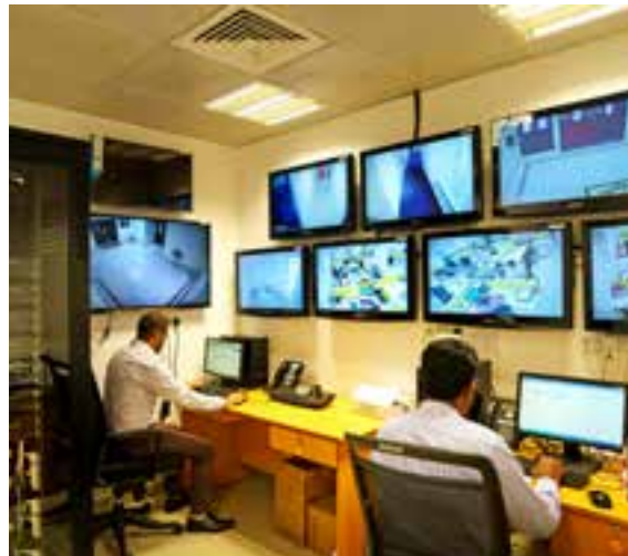
Central Surveillance & monitoring room
