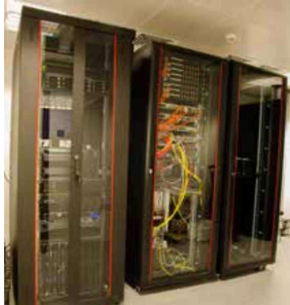
Head office Data Center
