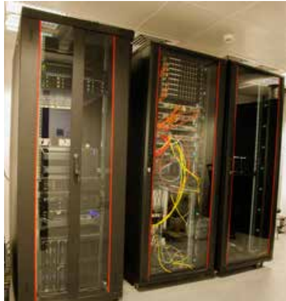
Head office Data Center
