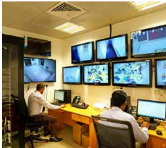
Central Surveillance & monitoring room
