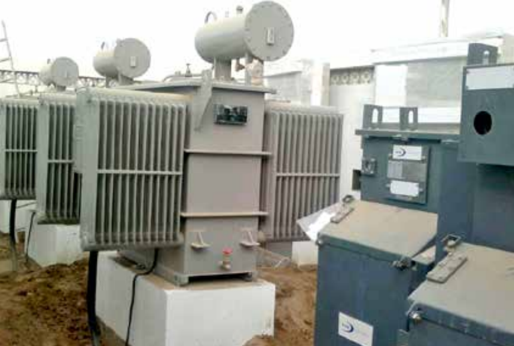
3 Nos of 1000 KVA substations with RMU
